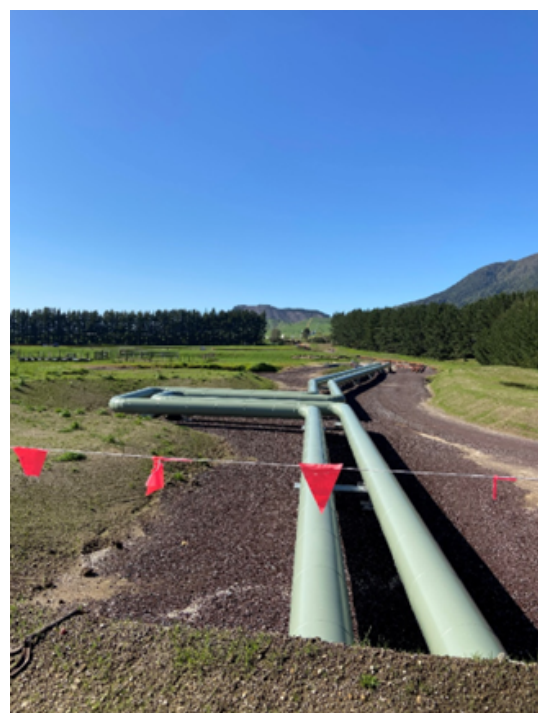
A photo from a Milford trip to the Tauhara Geothermal field. This is piping that takes steam from the drill well to the generation turbine hall to create electricity.
